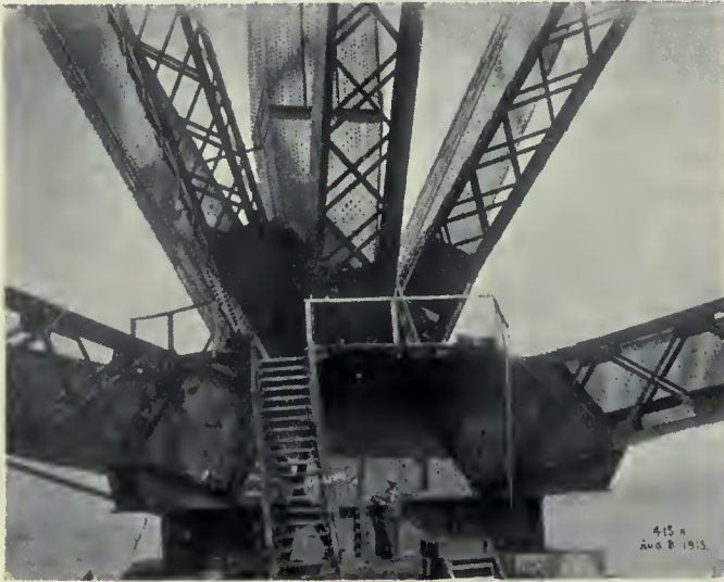
Fig. 2.—Intersection of ten members at the main shoe—Concentrated load on shoe about 55,000,000 lbs.
